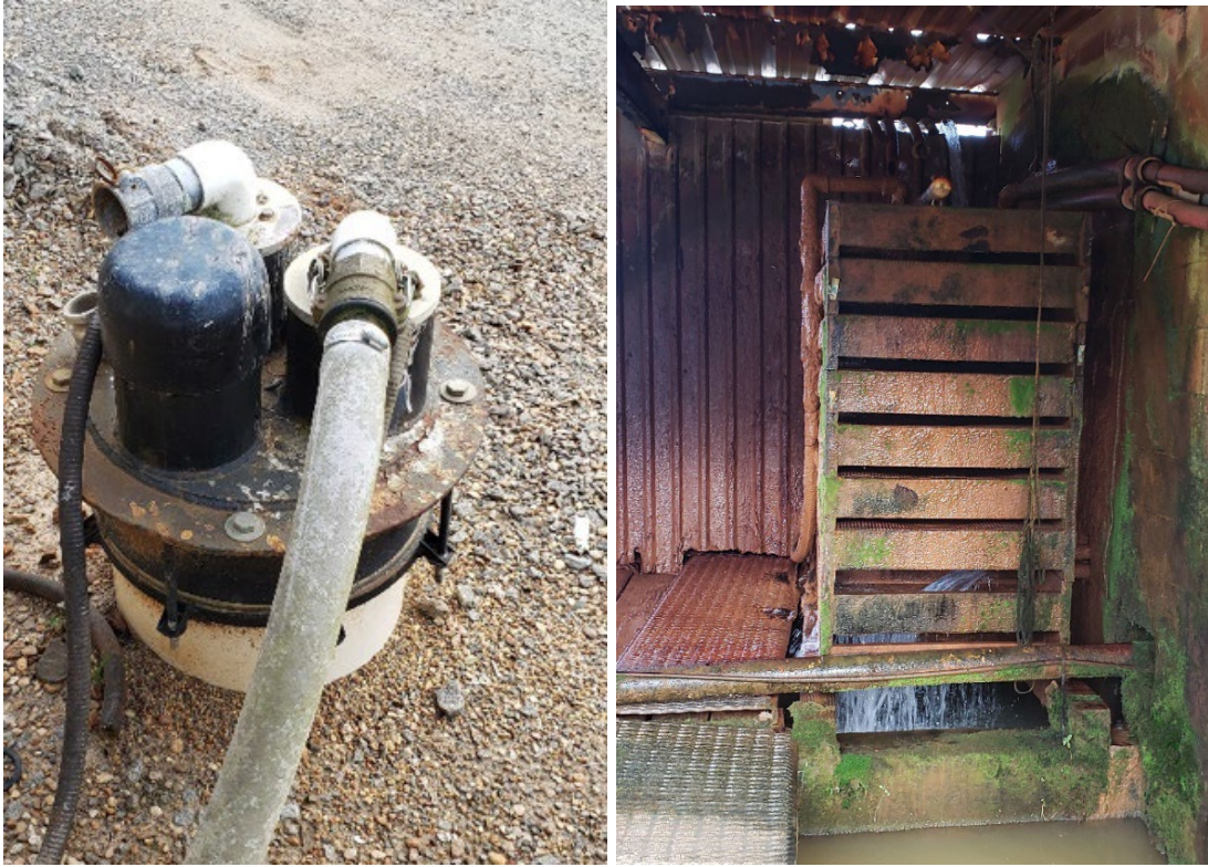
Figure 2a. Electrical pump located on top of the well. Figure 2b. Pit or aeration tower for releasing carbon dioxide.
