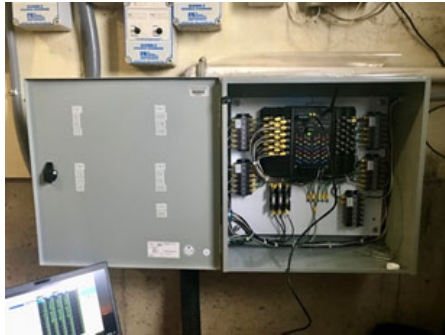
Figure 1. Electro Industries Shark MP200 multifunction energy meter installed at the main electric panel of the IGEM Farm.
