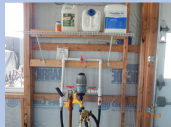
Figure 21. Examples of surfaces that should be sanitized and sanitizer installation
